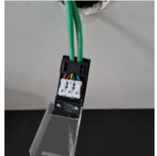
Example: looping of "low smoke" cable for public buildings
